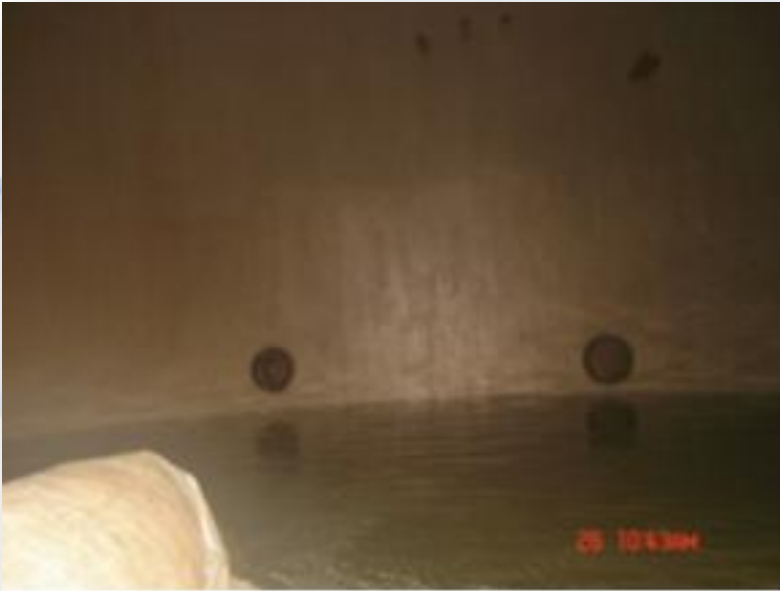
Check of Biogrowth and mold in tanks and pipes
